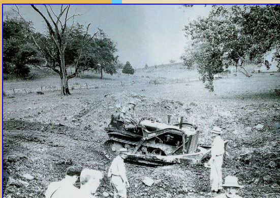
Fig. 2. Onset of 1954 bulldozer work at Lower Blue Lick. This search for “big bones” lasted a month and resulted in many important discoveries. Picks and shovels were used, and it seems that no sieving was done.
