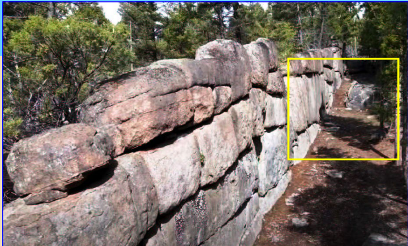
Fig. 1. A small portion of Sage Wall near Butte, Montana. The wall extends further in both directions. The part highlighted in yellow is the area represented in Fig. 2 below (which is Fig. 11 in Part 4 last issue, PCN #86 , Nov-Dec 2023). Photo: Christopher Borton.
