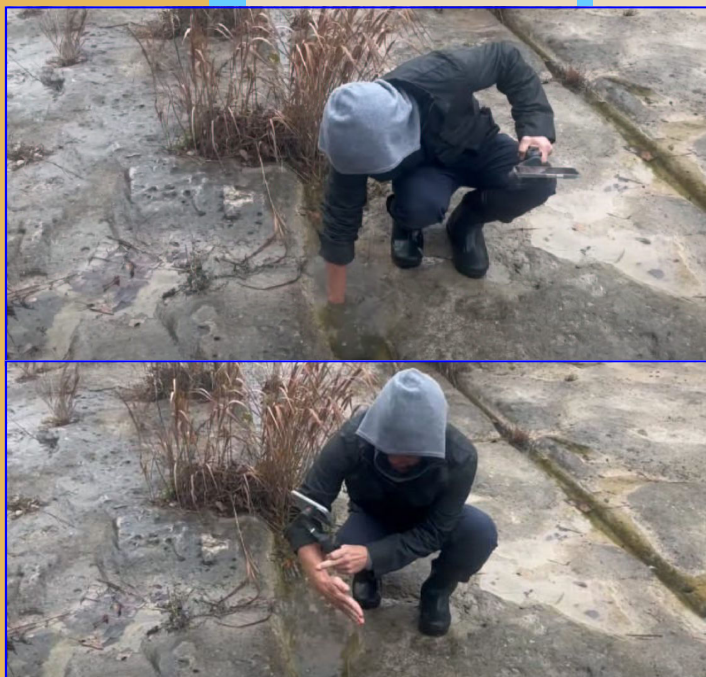
Fig. 3. Top: Kyle cleans out an Austin rut for a quick measure of its depth. Bottom: Quick check shows the rut is 10-12 inches deep. This would certainly be a rough track for anything other than state of the art modern wheel consistencies to ride in. Photos by Michael Collins.
